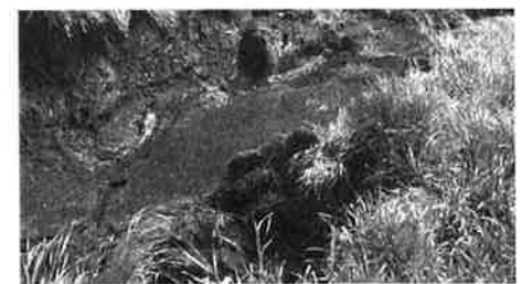
Gully erosion from May storm event, fixed with drop inlet.
